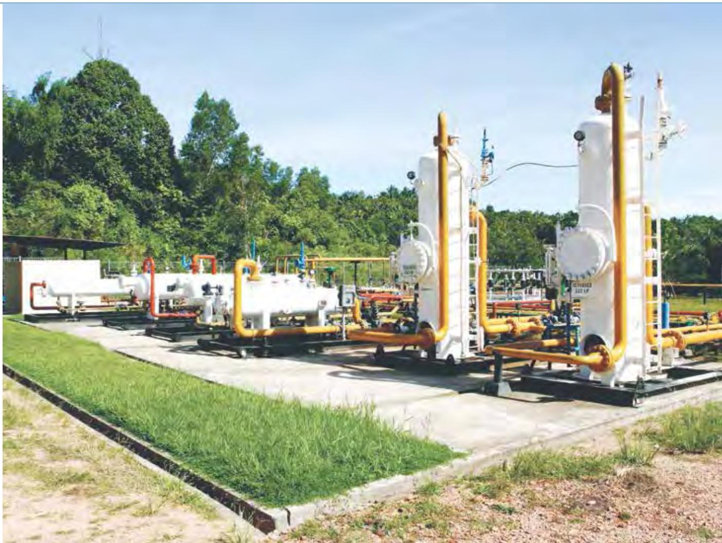
▲ Fasilitas pemrosesan dimana minyak dipisahkan dari gas di Blok Tarakan, Kalimantan Utara A processing facility in which oil is separated from gas at the Tarakan Block, North Kalimantan
