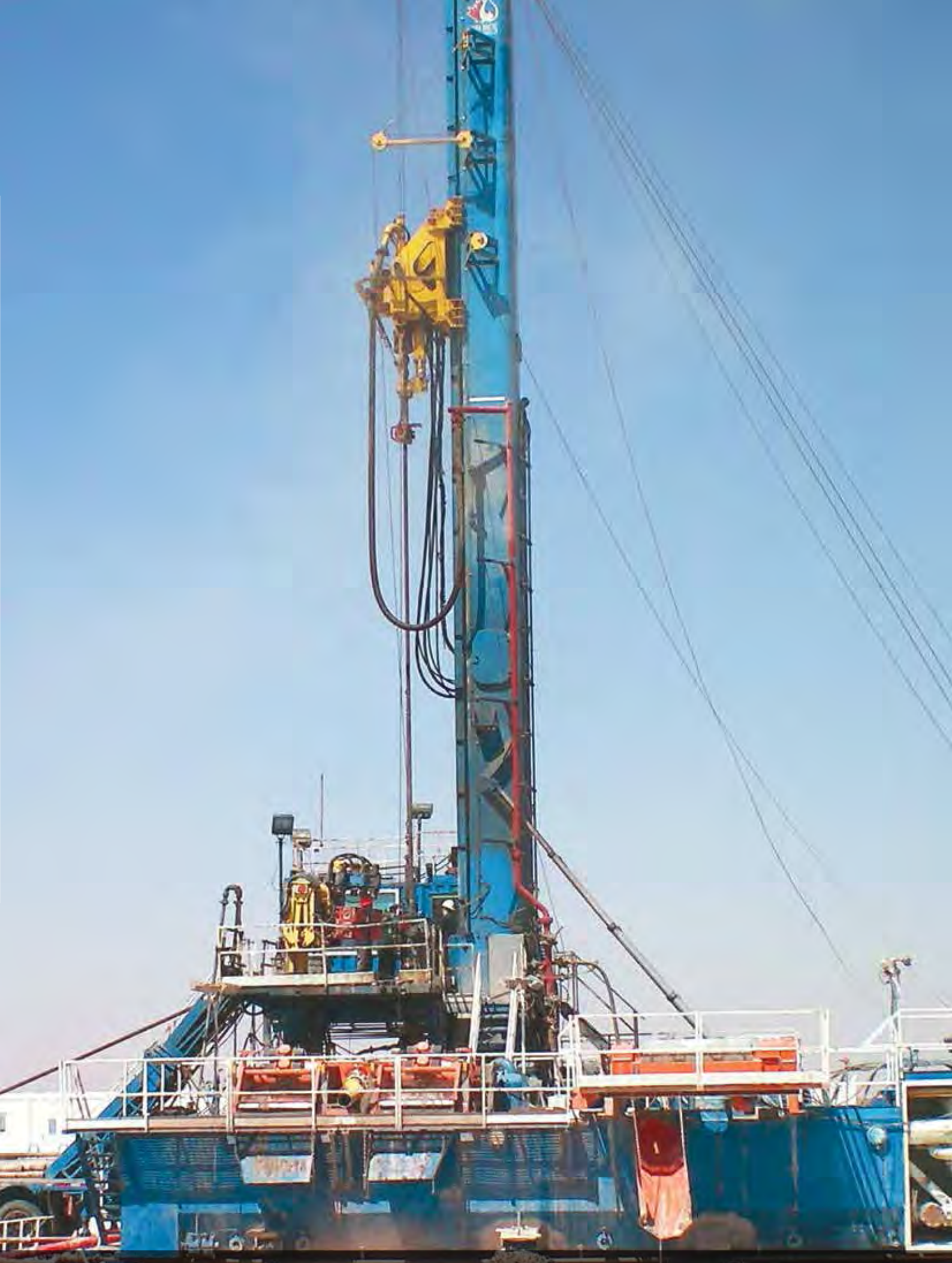
Fasilitas anjungan pengeboran yang sedang bekerja di salah satu blok Perseroan di Tunisia An onshore drilling rig facility in operation at one of the Company's blocks in Tunisia
